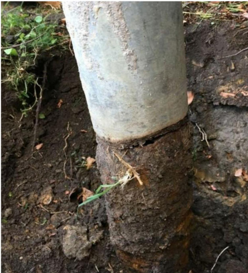
Typical corrosive damage to a galvanised steel pole.
