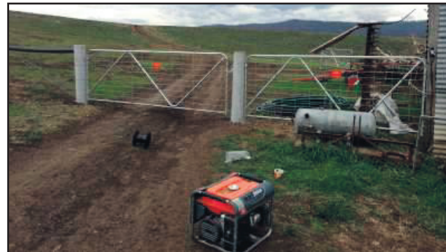
Titan strainer and gatepost section under construction using standard tools and equipment.
