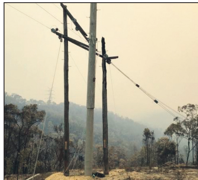
A two-part Titan pre-installed ready for a later change-over remained unscathed after a bush fire went through the site, December 2019.
